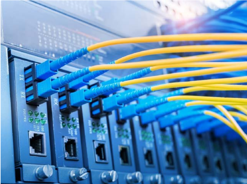
Figure 8: The hundreds of thousands of data centre servers, or nodes, are connected by optical cables. Credit:kynny/Istock
